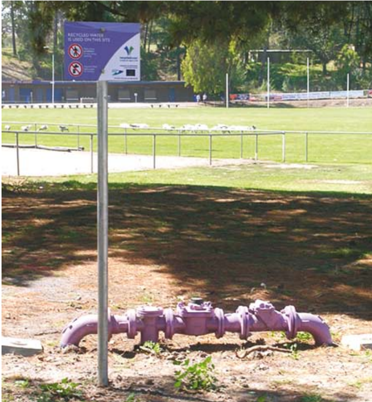
■ Salesian College Oval's recycled water meter
