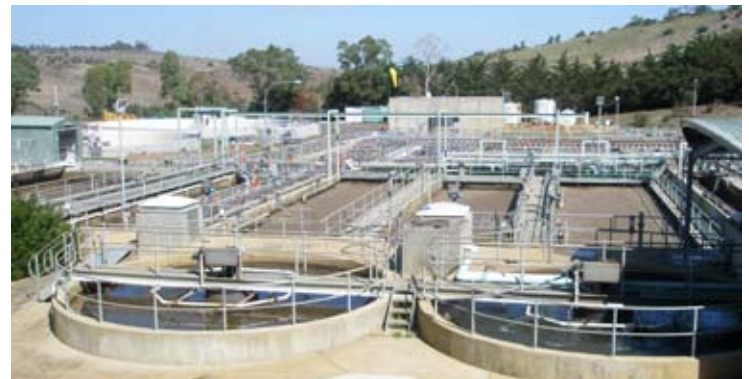
Above: Sunbury Recycled Water Plant.
