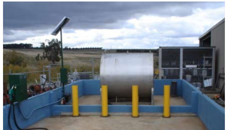
The biodiesel tank, with a new solar panel and pump, at Western Water's Gisborne Depot.
