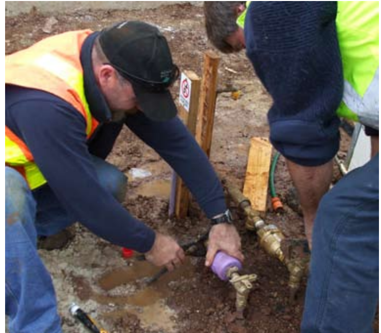
A purple meter for Class A recycled water is installed by a Western Water crew at a new house site at Eynesbury.
